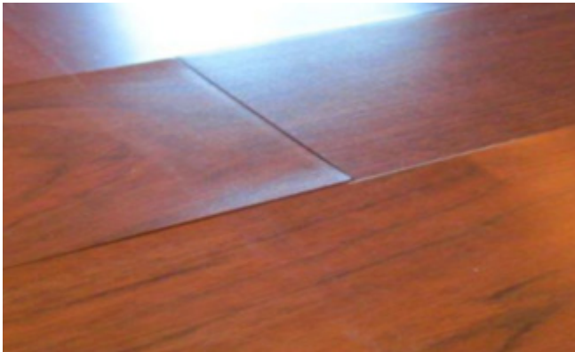
Dry cupping (boards deform and lift at edges) Cause: Improper humidity levels
