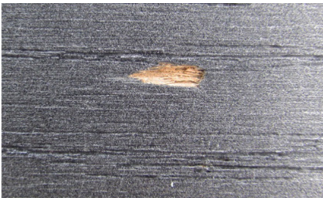
Scratches and chips in floor surface Cause: Trade damage
